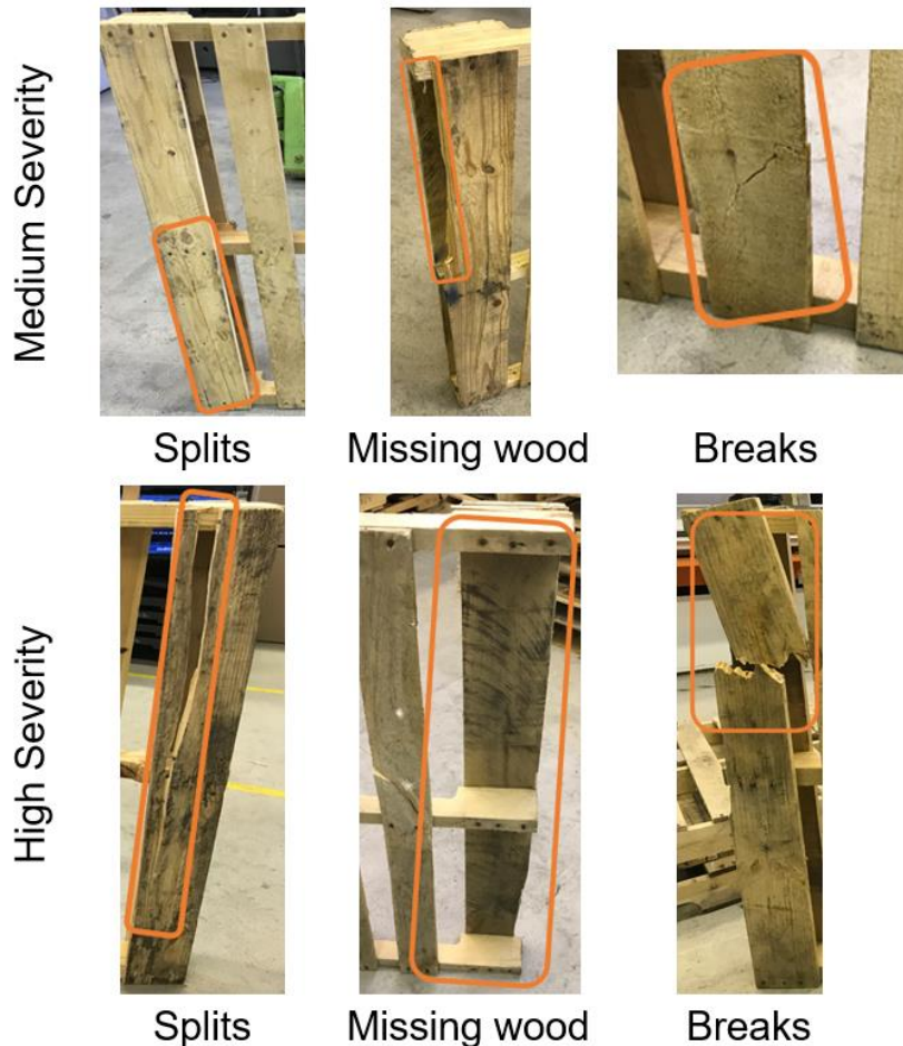
Fig. 3. Representative picture of splits (left), missing wood (middle), and breaks (right) based on severity scale
